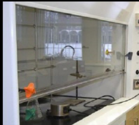
Acid Digestion Hood with Polycarb Sash & Plastic Ducting
